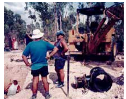
Jabiru, 1993 – New Borefield Rising Main
